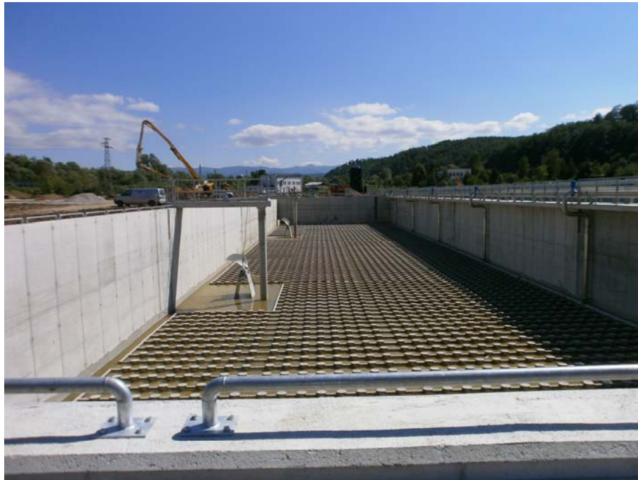
Figure 1: Basin overview - CYBERFLOW ® - Accelerators & iDISC ® - Membrane Aerators
