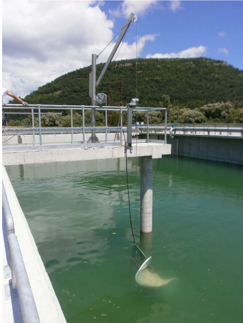
Figure 4: CYBERFLOW ® - Accelerator installed
